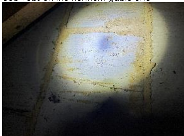
Photo 6 – bat droppings recorded in cobwebs on the northern gable end
