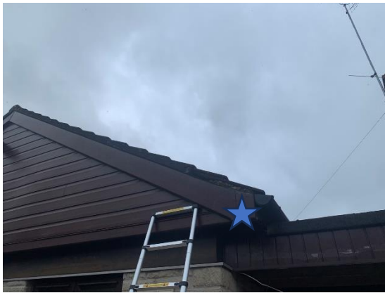
Photo 17 Location of gap into PRF on east elevation of building
