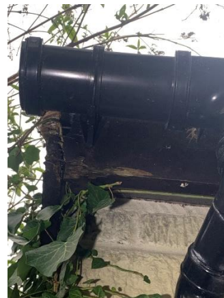
Photo 22 Damage to soffit on south west elevation
