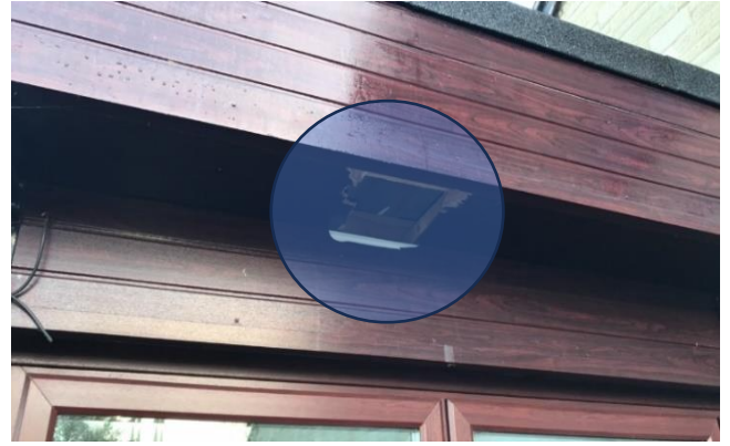
Photo 16 Damage to soffit, creating potential access gap into PRF1
