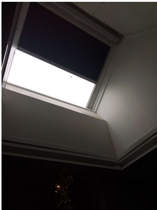
Velux In Area FR1 & FR2 Velux X 3 will need to be replaced, very close to the end of life.
