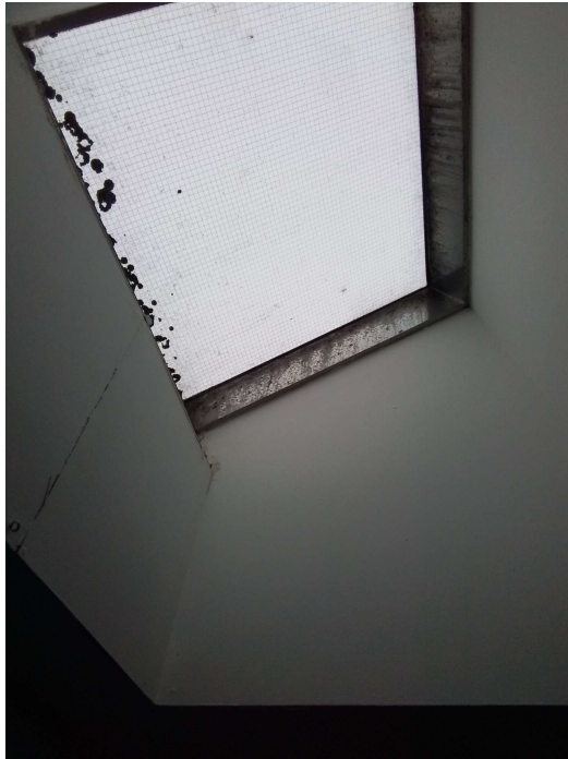
Skylight X 1 To Be Replaced In Area FR1 Skylight end of life.
