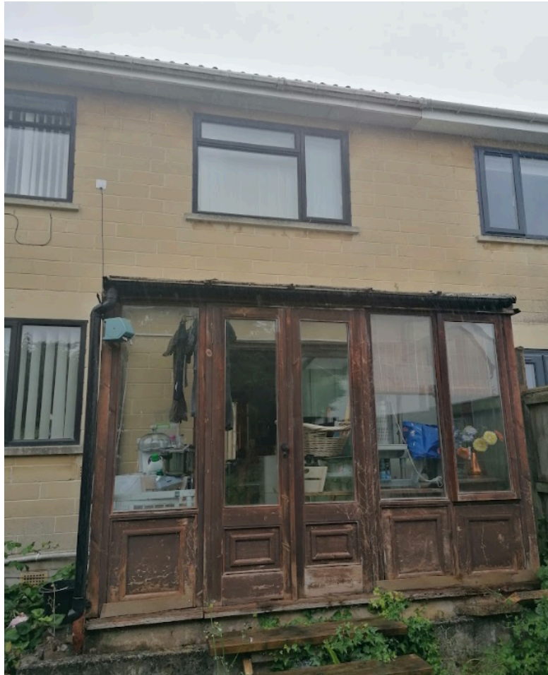
View from rear garden of poor performing existing rear extension
