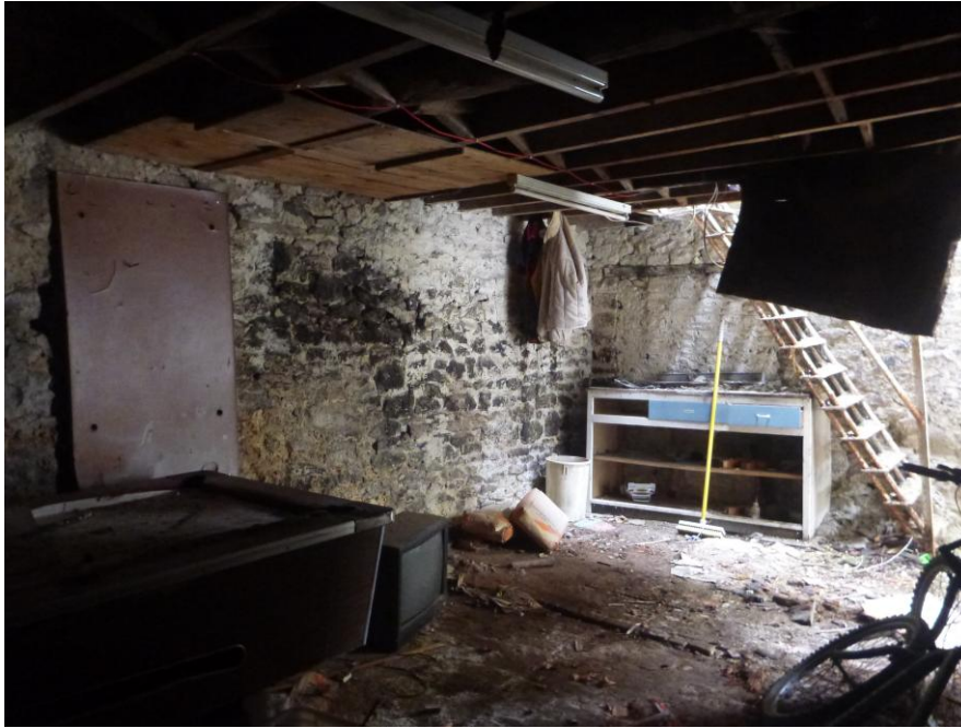
Fig 6: Part of the roof has blown off, allowing daylight to penetrate the upper floor of the barn. The intermediate floor prevents light spill into the ground floor.
