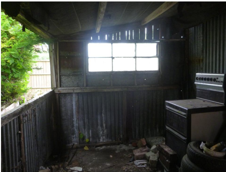
Fig 9: A missing window on the north face of the single storey lean-to.
