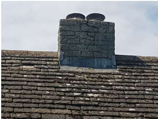
Photo 7: B1 - A missing tile on the rear north-east facing roof aspect
