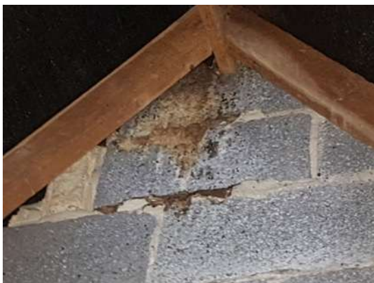
Photo 9: B1 - Grease staining near the apex of the north-western gable end wall.
