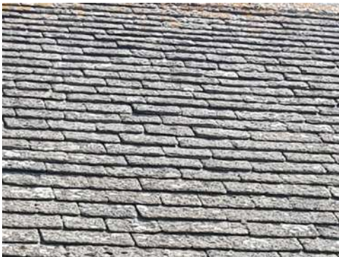
Photo 5: B1 - Low number of suitable gaps present beneath the imitation stone tiles.
