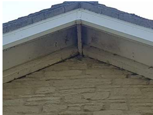
Photo 6: B1 - gap at roof edge, apex of the north-west facing gable end.
