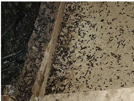
Photo 12: B1 - droppings were present throughout the loft void.
