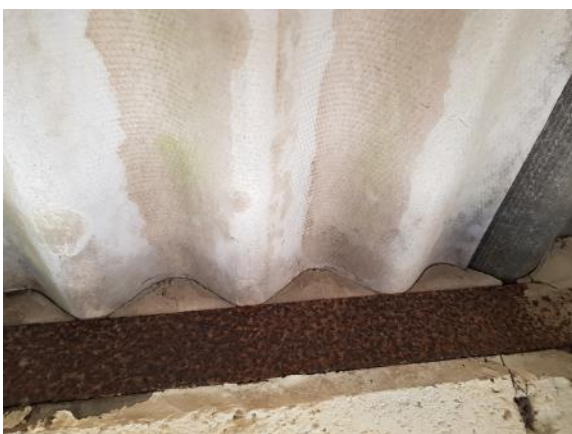
Photo 11: Junction between roofing sheets at the eaves filled with mortar.
