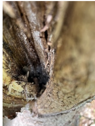
10: View into knot hole cavity.
