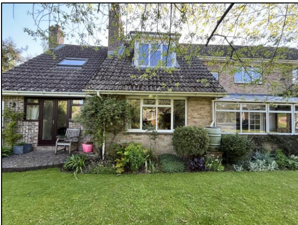
West elevation showing leaking dormer and velux to be replaced
