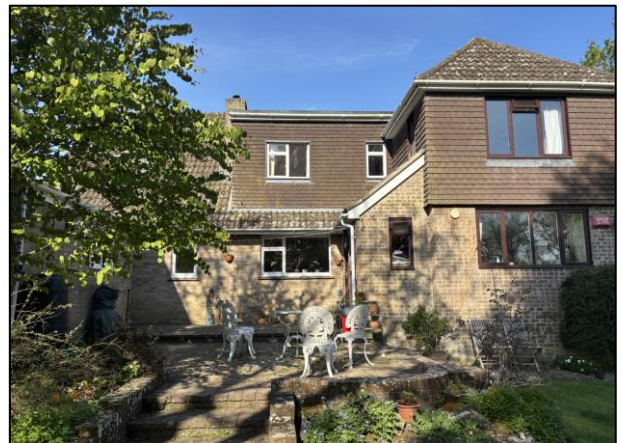
East elevation showing box dormer and areas of tile hanging to be replaced
