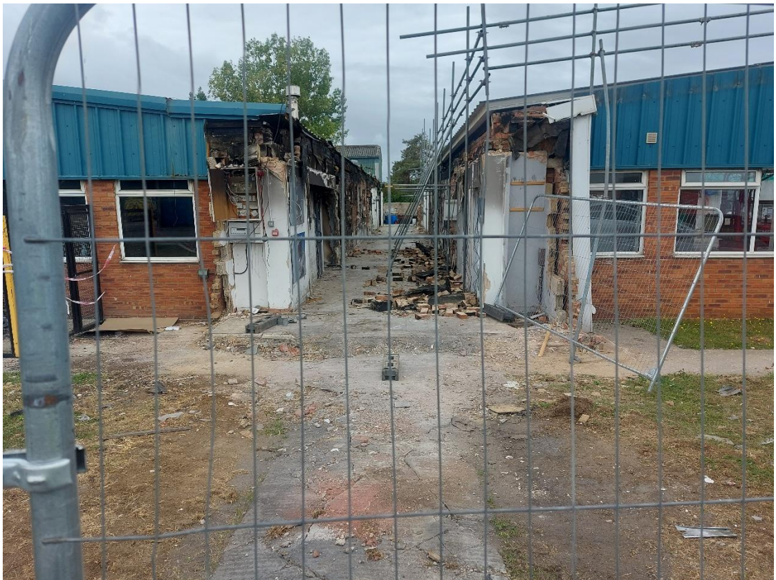
Figure 5: View of fire damaged section of building
