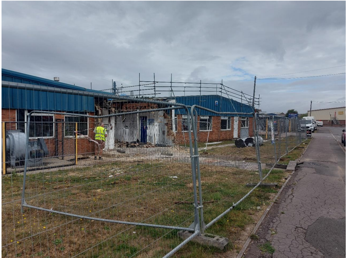
Figure 5: View of fire damaged section of building from Porte Marsh Road
