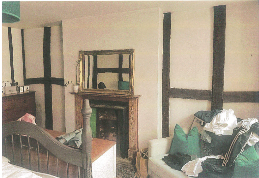
Figure 13 The west wall of the front first floor bedroom.
