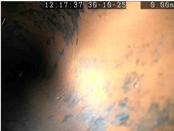
b70e7b46-f2e4-482a-9a24-d8bf7599823.png, 00:00:06, 0.00 m Start node, manhole, reference: I/C1
