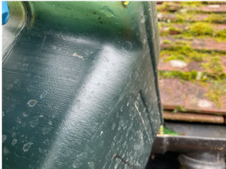
Photograph of dye test undertaken
