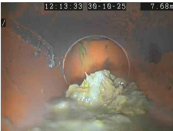
a9c59574-7c2b-472e-8a7d-523843b1fb4d.png, 00:01:34, 7.68 m Attached deposits, grease from 5 o'clock to 7 o'clock, 15%
