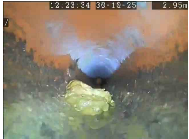
5c243ea2-1912-4433-8fbd-e34634534764.png, 00:00:15, 2.95 m Attached deposits, grease from 5 o'clock to 7 o'clock, 5%
