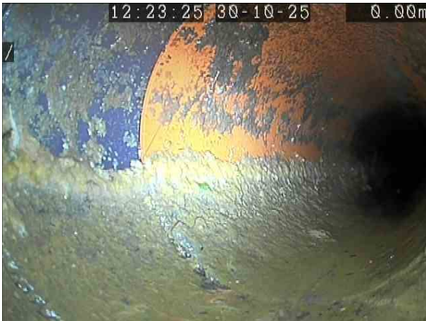
1fb41805-a1bd-419e-ae95-51c39206bae9.png, 00:00:06, 0.00 m Start node, manhole, reference: I/C2
