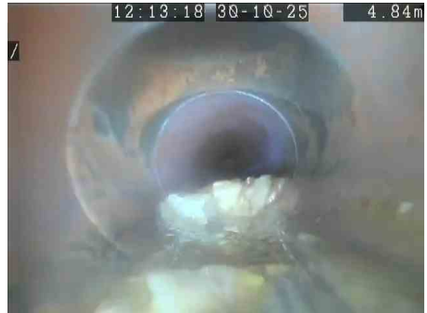
59199569-7f25-43fa-bdfa-235cc5e65efc.png, 00:01:19, 4.84 m Attached deposits, grease from 5 o'clock to 7 o'clock, 10%
