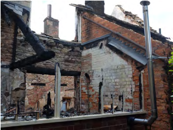
Fig.26 Charred roof trusses and flue from C20 range
