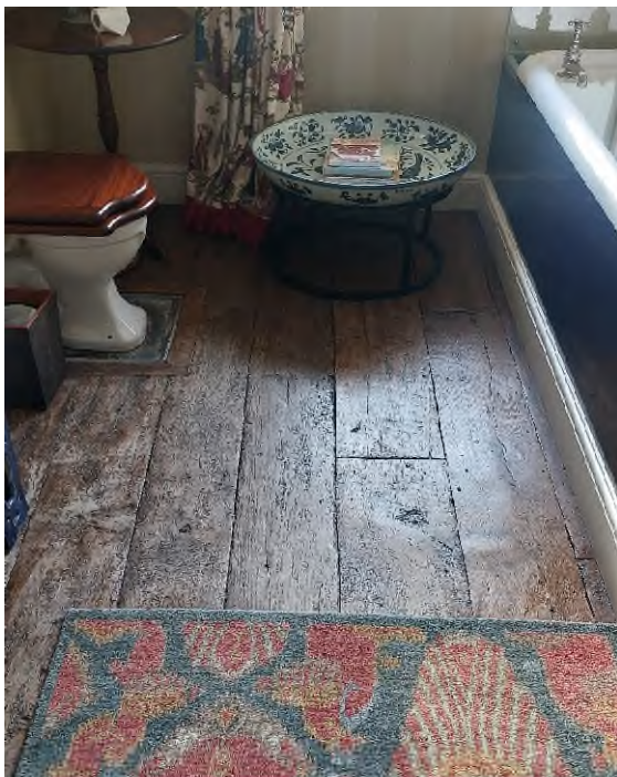
Photo 11 Bathroom B15. Reclaimed floor boards.
