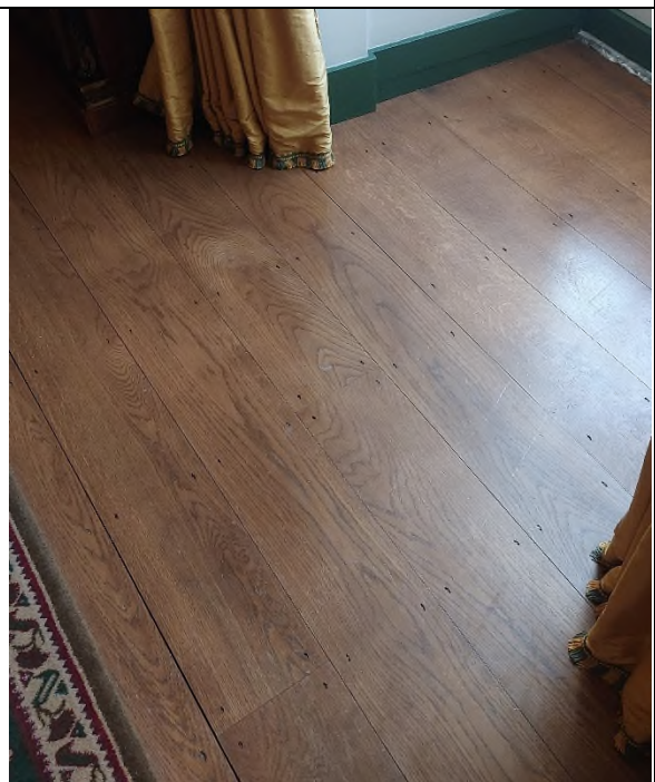
Photo 19 Large Smoking Room, B40
