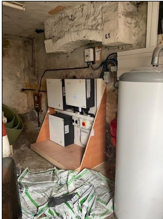
Picture 10: Equipment and batteries will link to existing system in the garage
