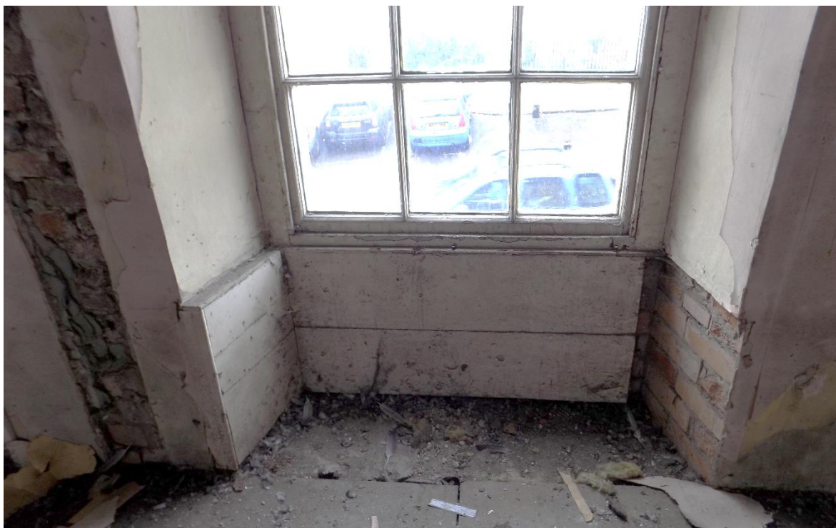
Fig.28: First-floor: Detail of third front-facing window from west, showing historic window seat truncated by false floor.
