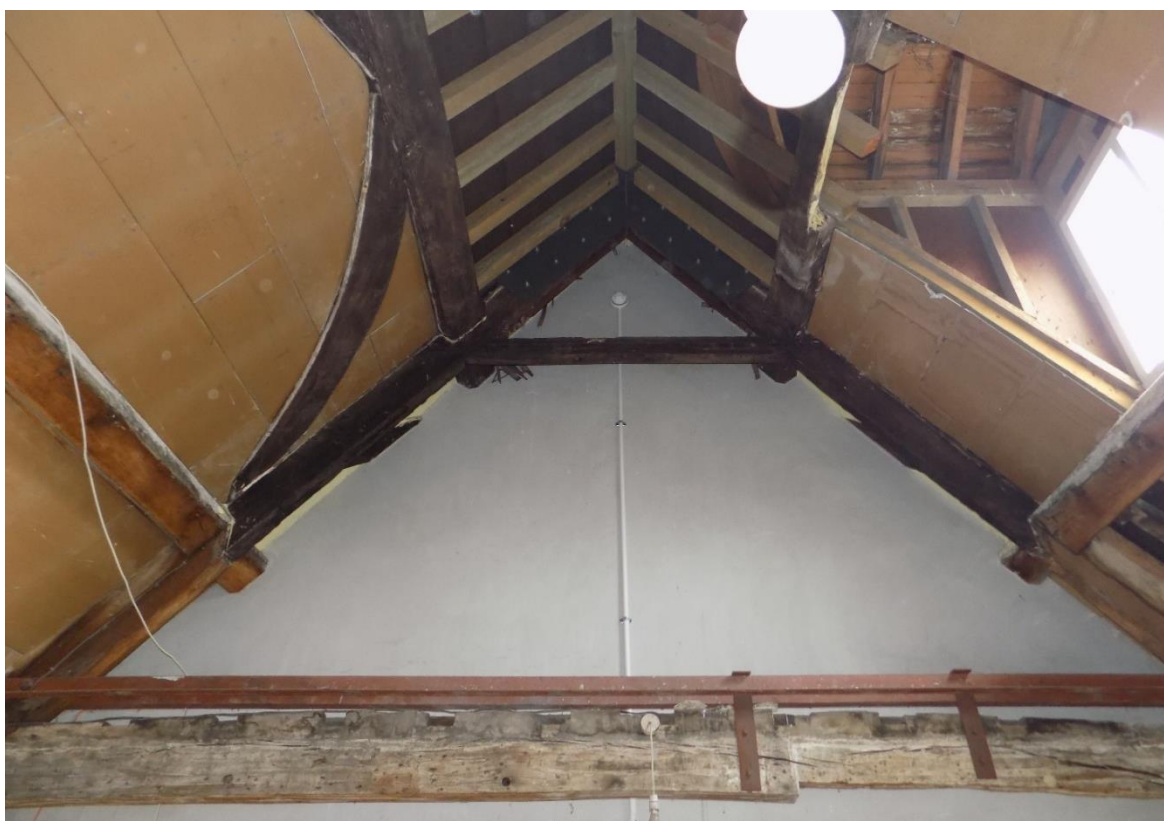
Fig.41 Attic view looking west, showing third tie from east notched for joists along its full length.
