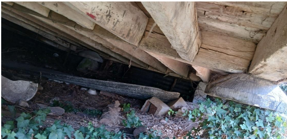
Figure 7 - Failed timber base structure
