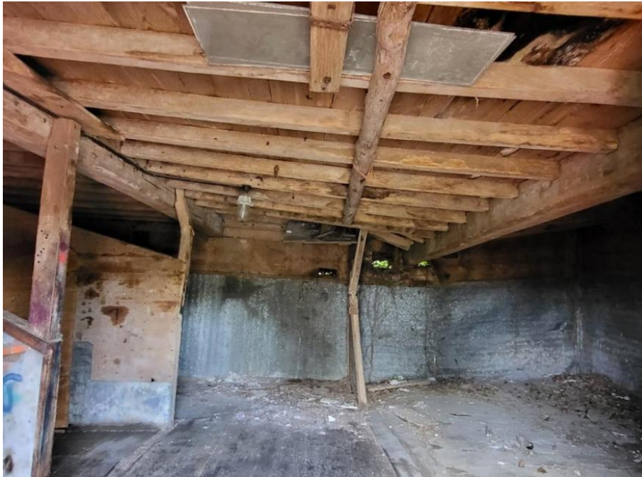
Figure 6 - Failed beam in small granary
