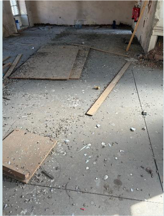
Considerable pigeon droppings and detritus covered the floor.
