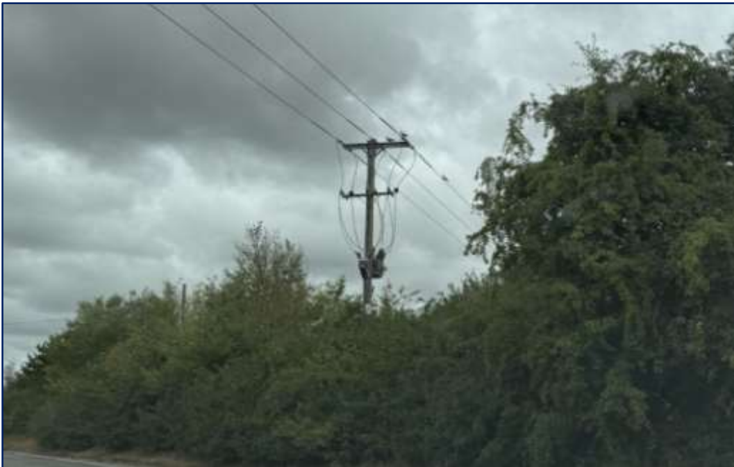
Figure 5: Existing switch gear to the south of Swindon Road
