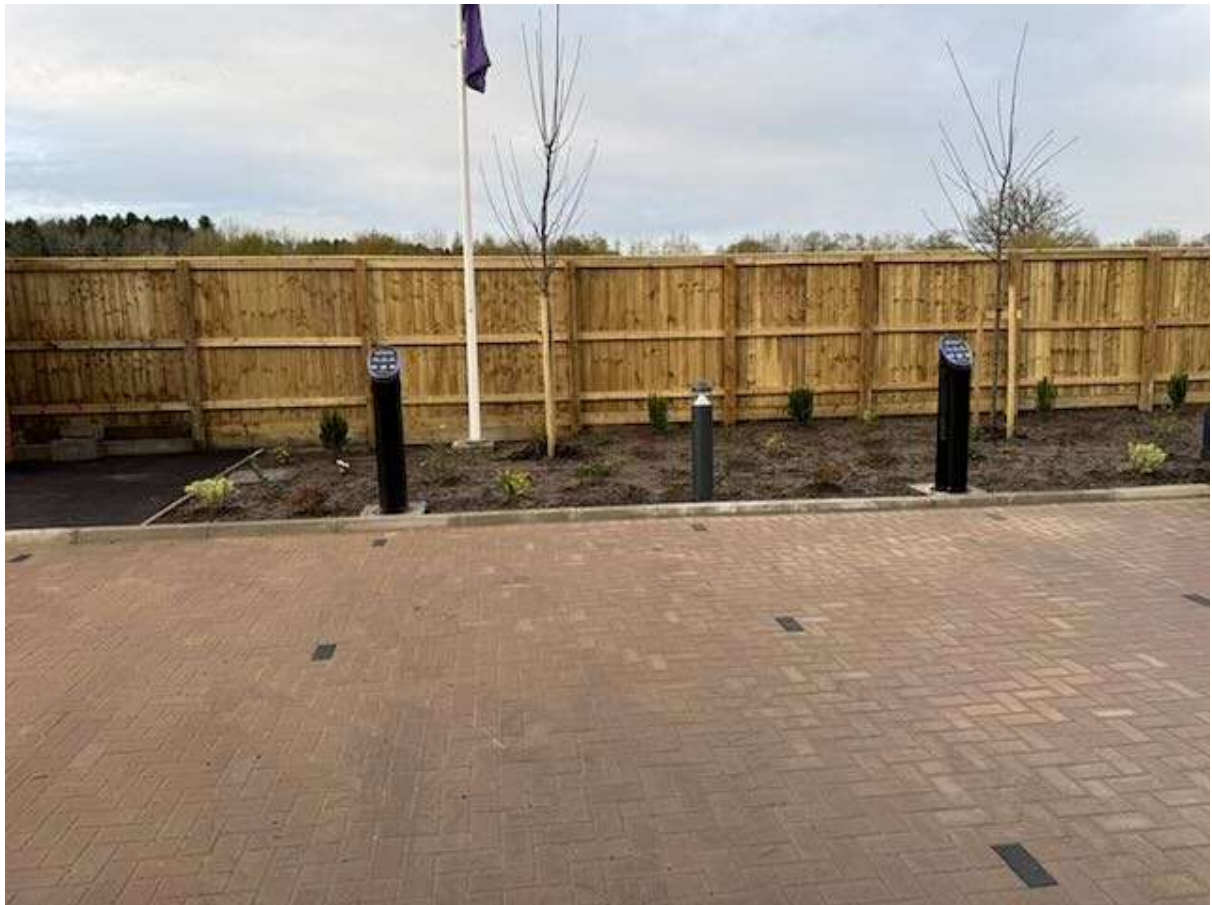
The 4 parking spaces with EV charging points.
