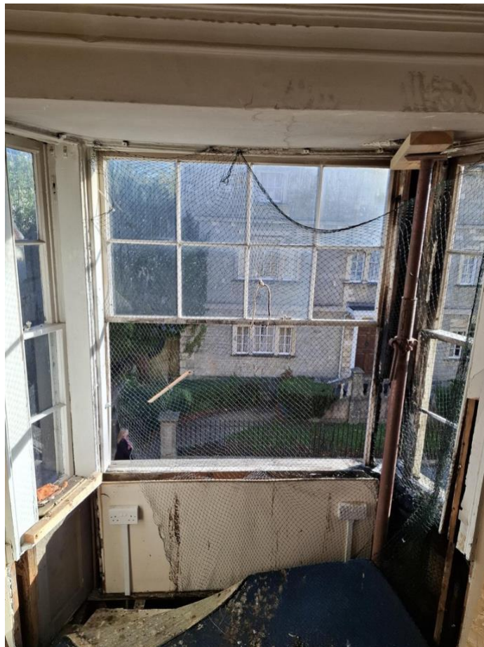
Photo (iii) – damage from fire internally
