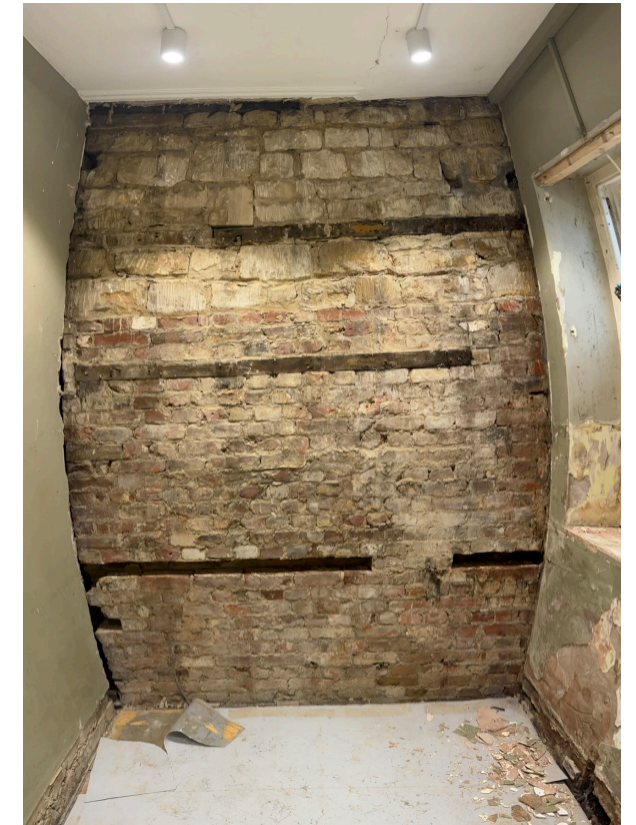
West elevation showing the lower inset timber rotted away
