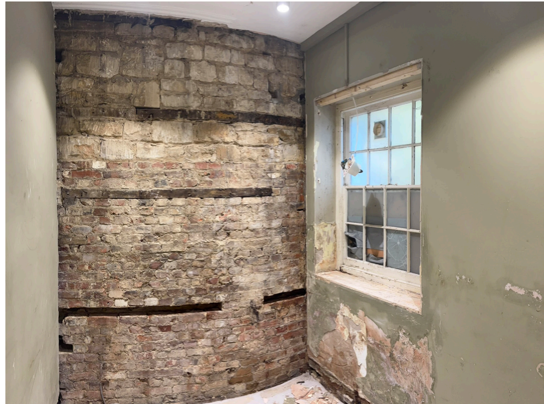
The west elevation with the original lath & plaster wall lining removed & north elevation with damaged plaster & window
