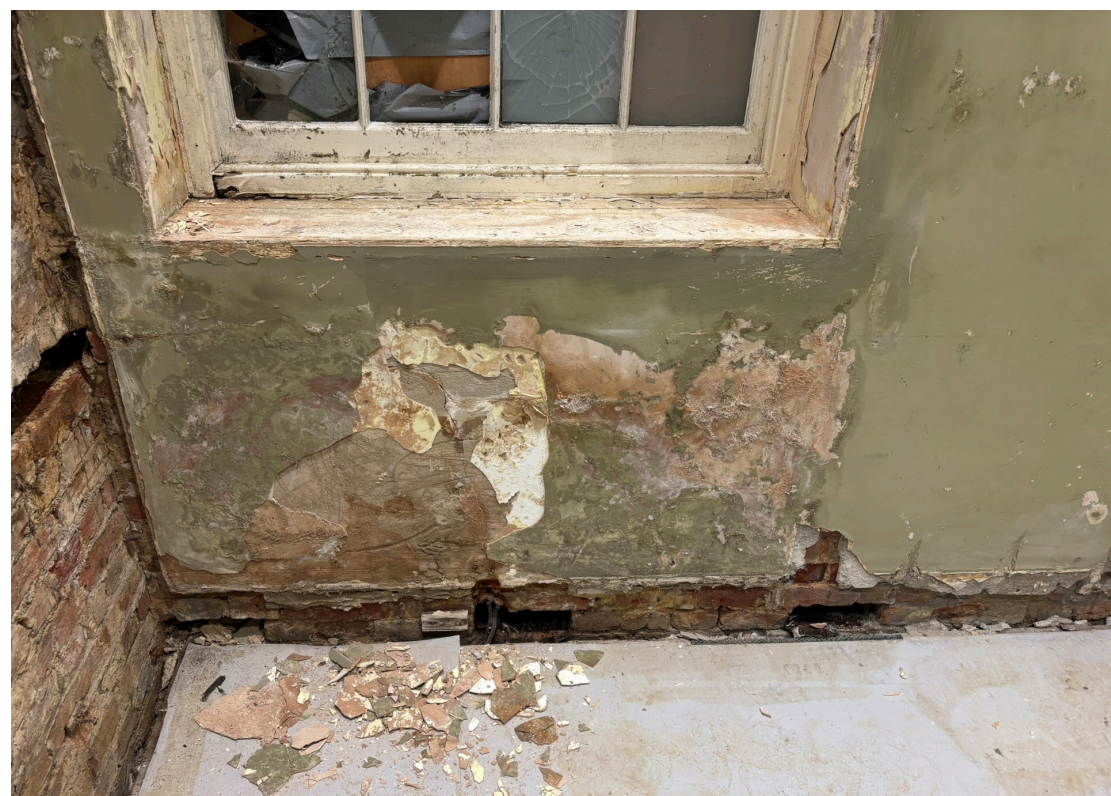
Low level existing bonding plaster damage beneath the north elevation window.
