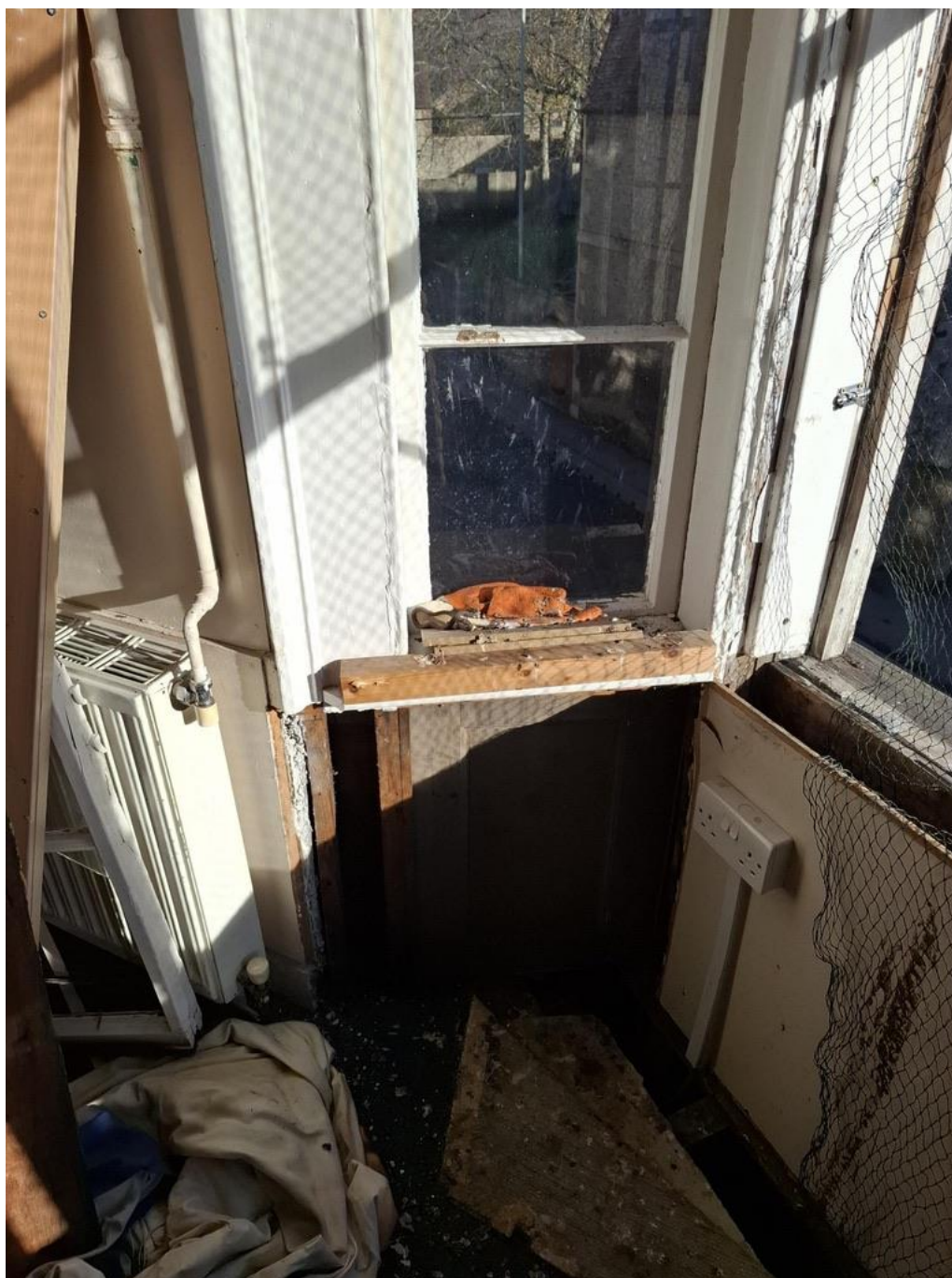
Photo (v) – timber panelling beneath window
