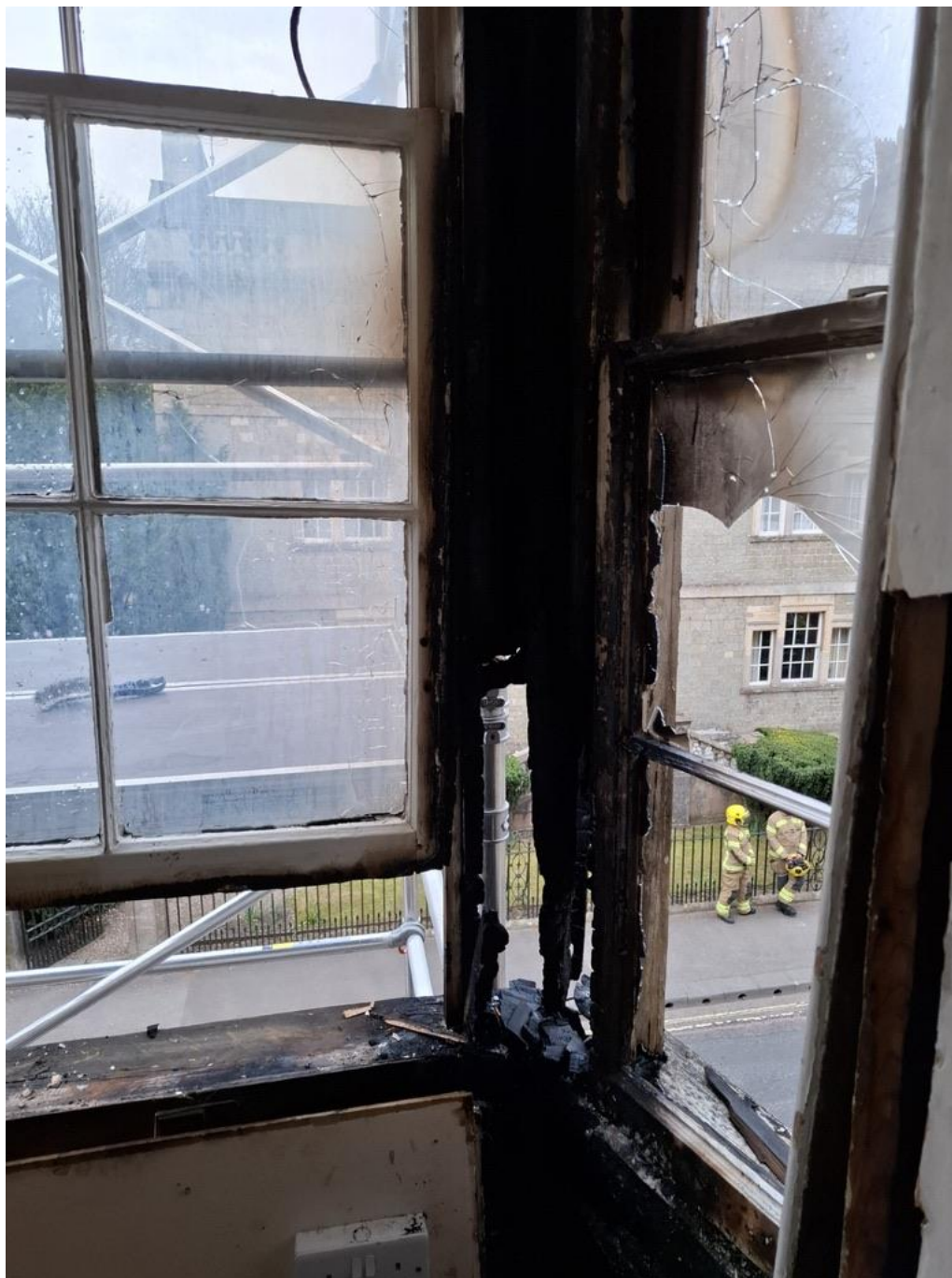
Photo (iv) – damage to timber box frame
