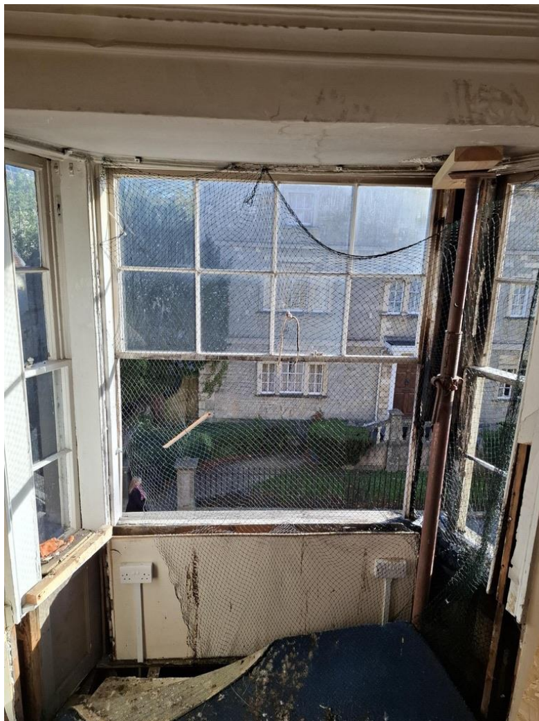
Photo (iii) – internal damage
