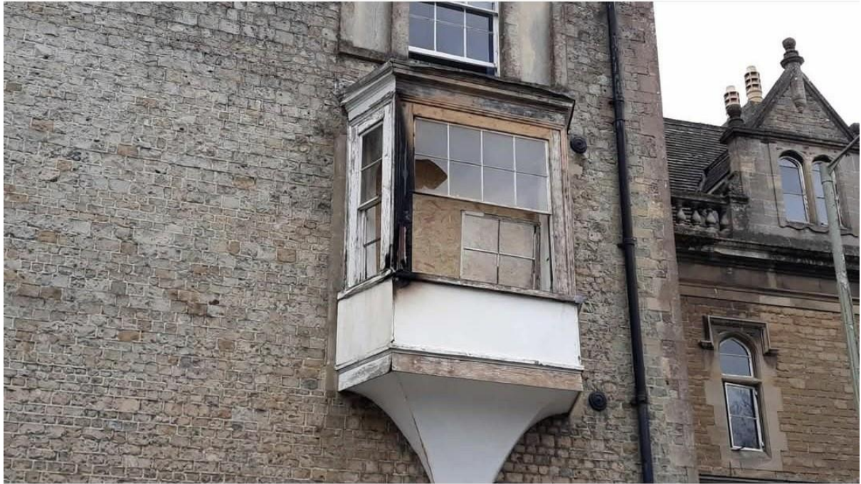
Photo (ii) – close up of damage to oriel window
