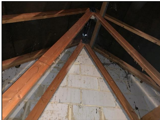
Photo 9 Loft void gable end with bat droppings
