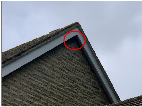
Photo 7 Southern soffit – bat roost entrance
