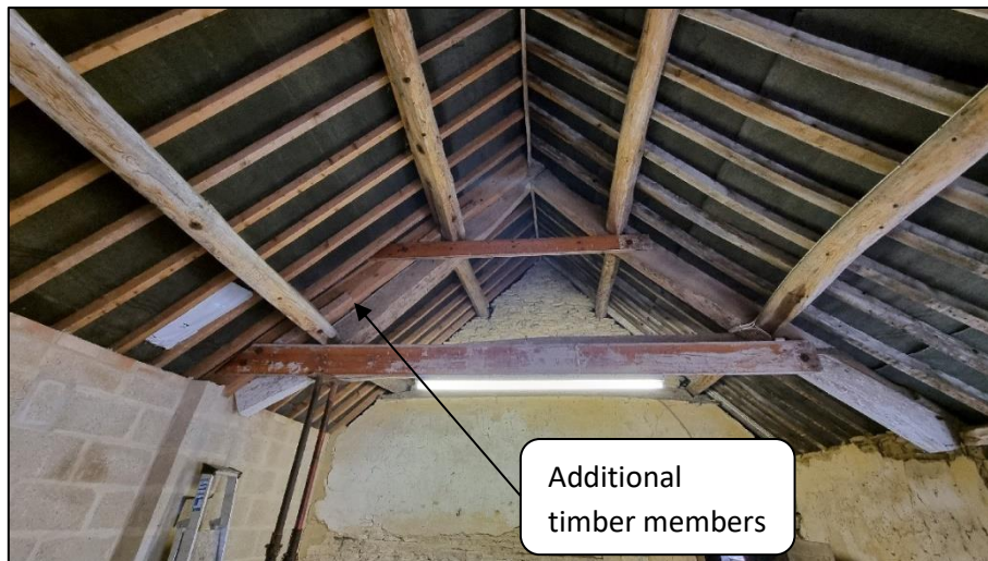
Photograph 6: Movement to the truss
