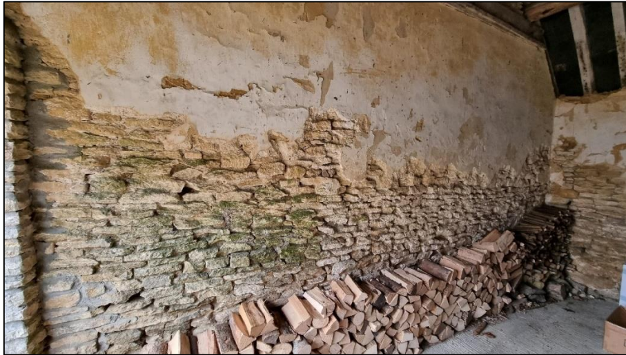
Photograph 4: Wall requires re-pointing
