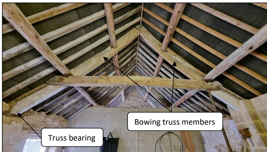
Photograph 5: Movement to the truss
