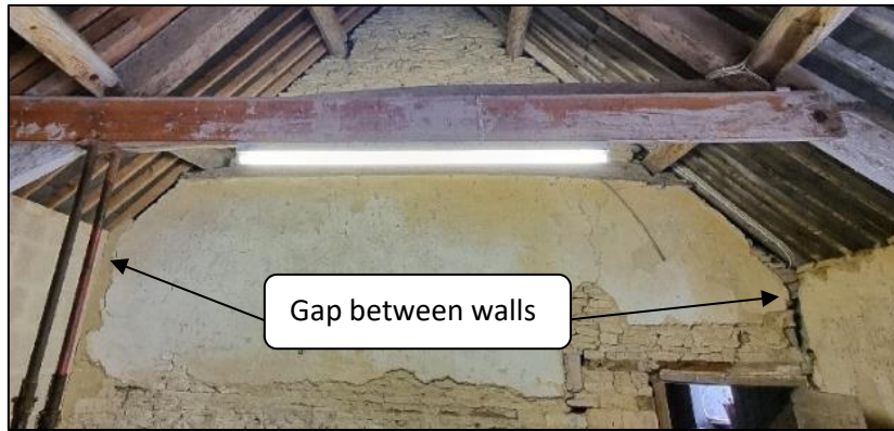
Photograph 8: Gaps between the internal and front & rear walls
