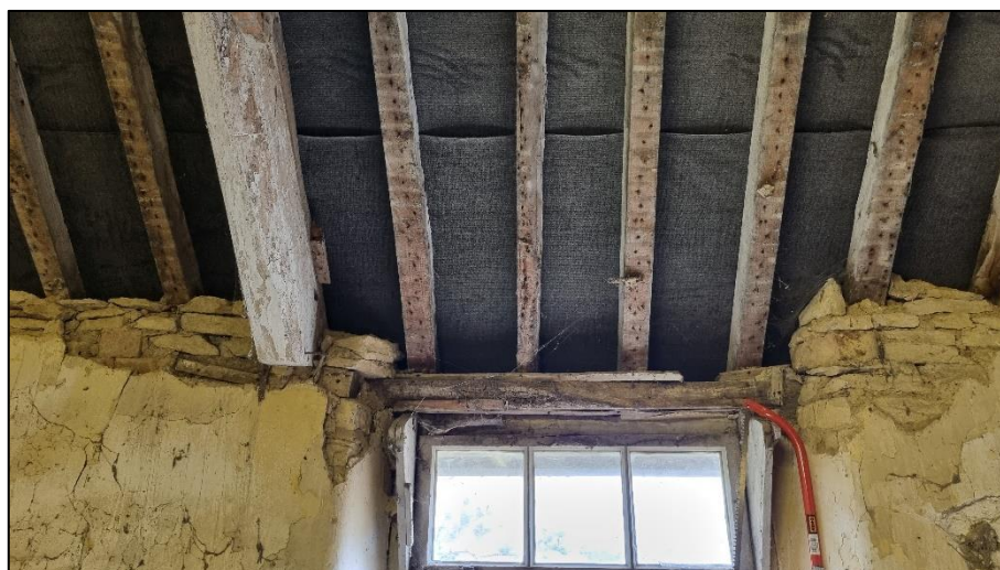
Photograph 7: Deterioration on timber lintel and masonry wall
