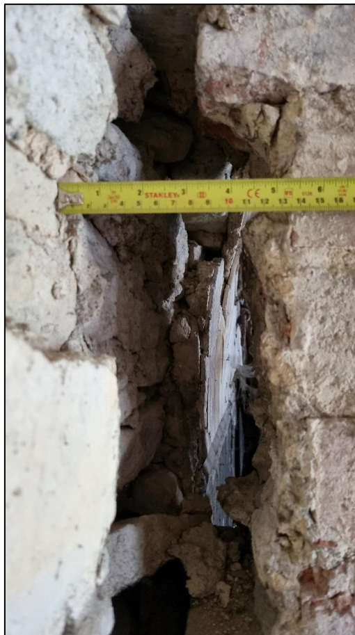
Photograph 9: Gap between the internal and front & rear walls
