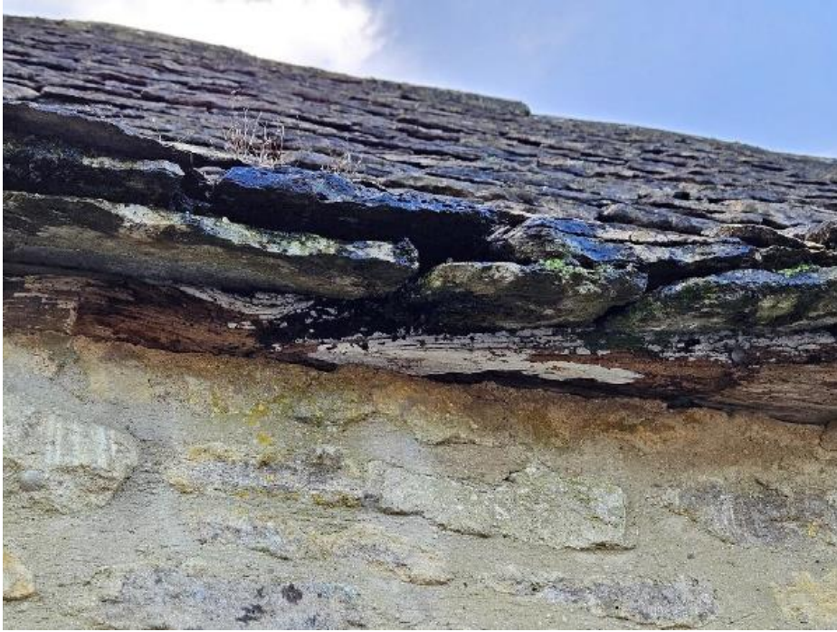
Fig.10 Damage to the wall plate due to water ingress at the eaves
