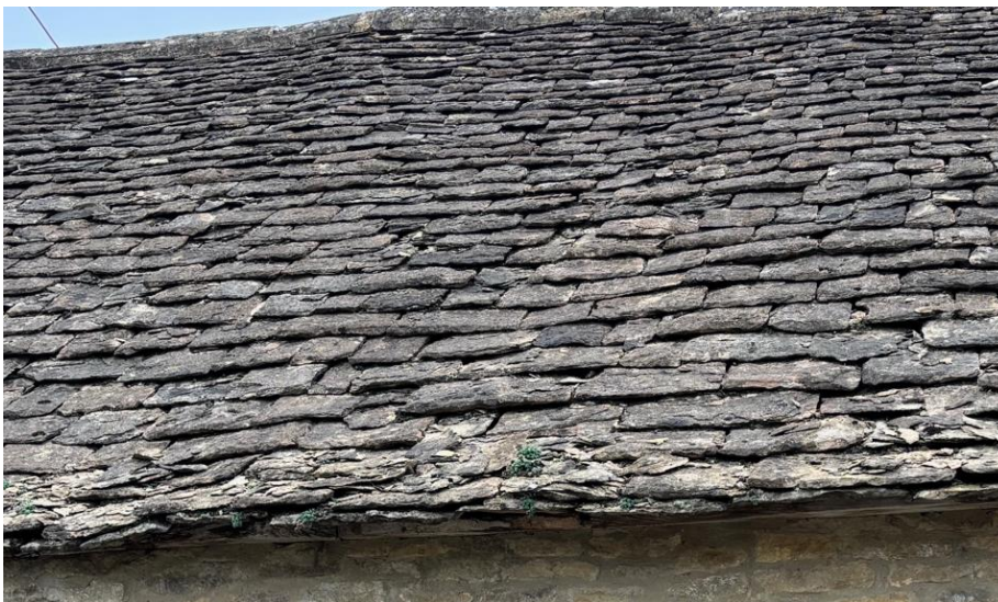
Fig.9 Close-up of the stone tiles showing delamination and slipped tiles
