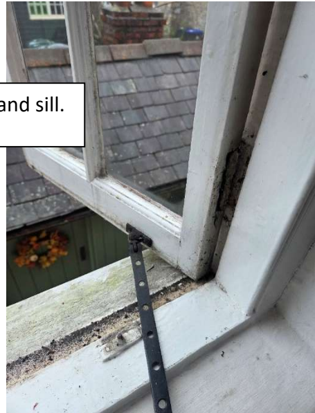
W1 – hinge and sill damage
