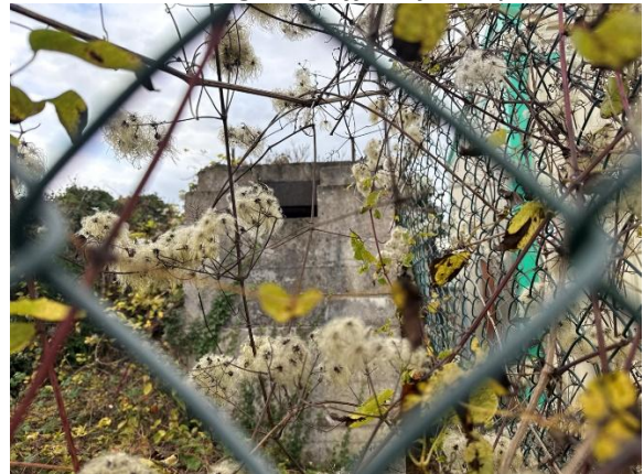
Photo 10 Offsite breezeblock structure (showing void on northwest façade) (B3)
