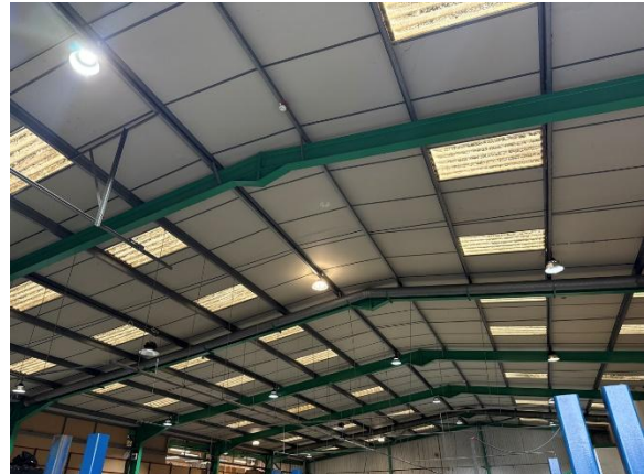
Photo 8 Interior lighting offsite factory (B2)
