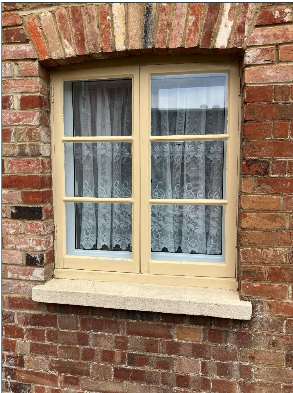
Figure 12 – Non-original single glazed side hung timber casement window with secondary glazed unit fitted to internal reveal.
