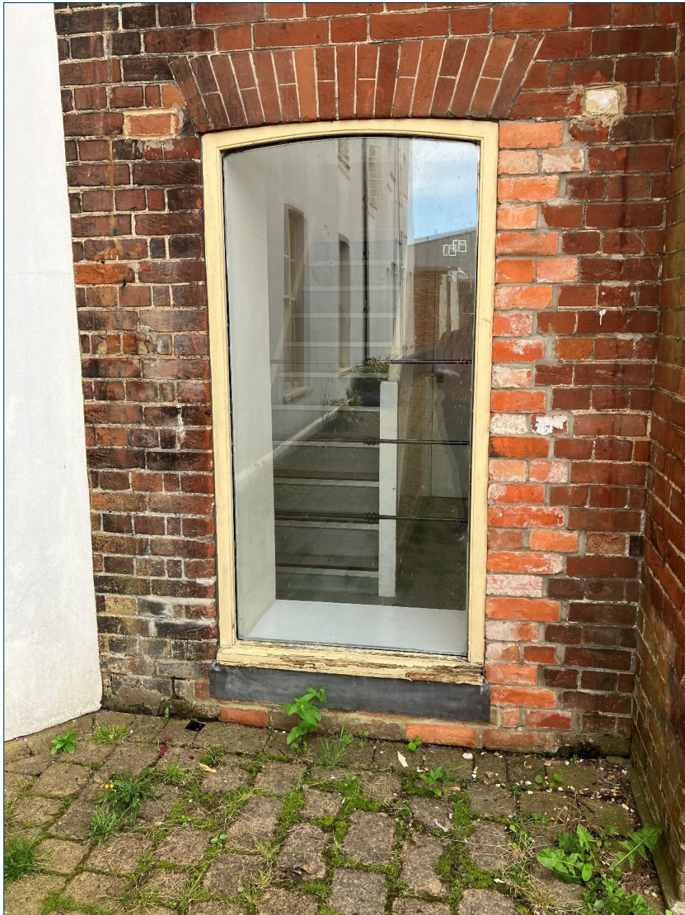
Figure 9- Example of non-original timber double glazed single fixed pane window installed to stairwell.
