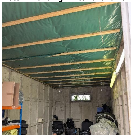
Plate 3: Building 1 PRF – gaps under barge boards
