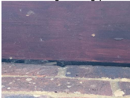
Plate 6: Building 2 PRF – missing mortar
