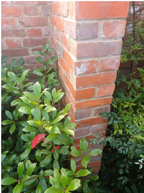
Wall – buttress added following planning approval in 2016
