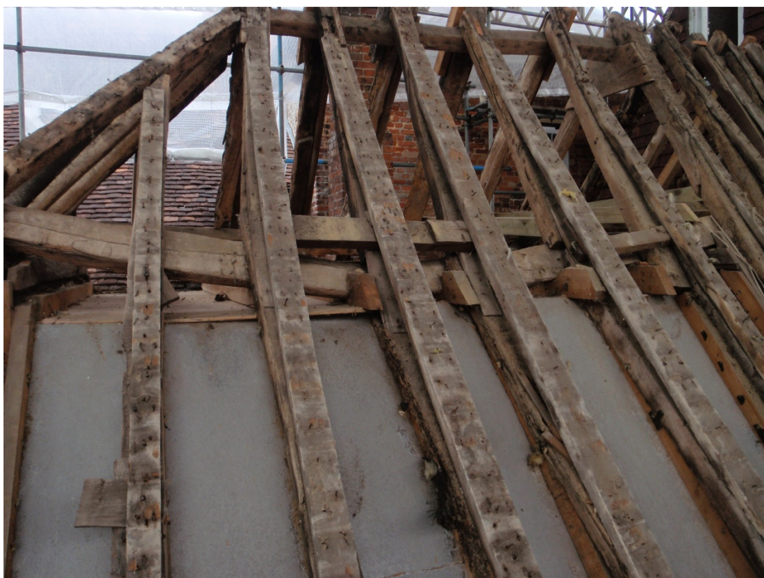
Fig 2 Fractured purlin and poor rafters.
