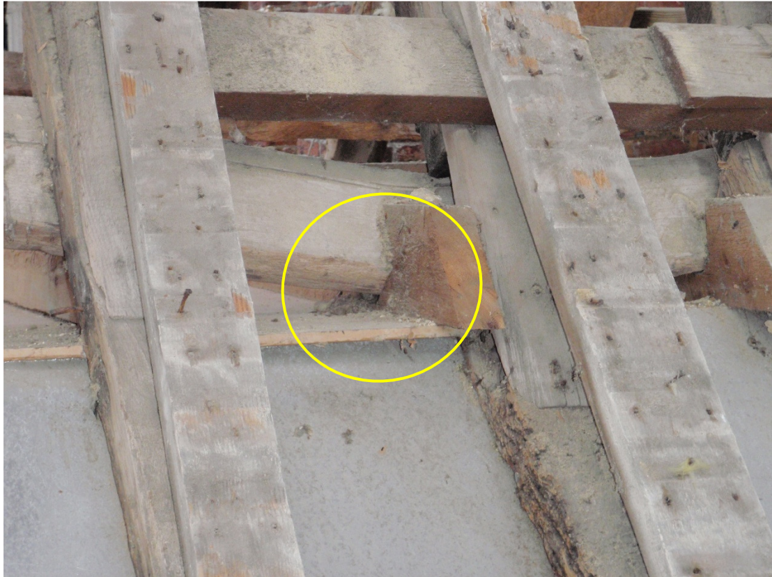
Fig 3 Minimal amount of timber remaining to ceiling joist cut to suit purlin, which is fractured in any case.
