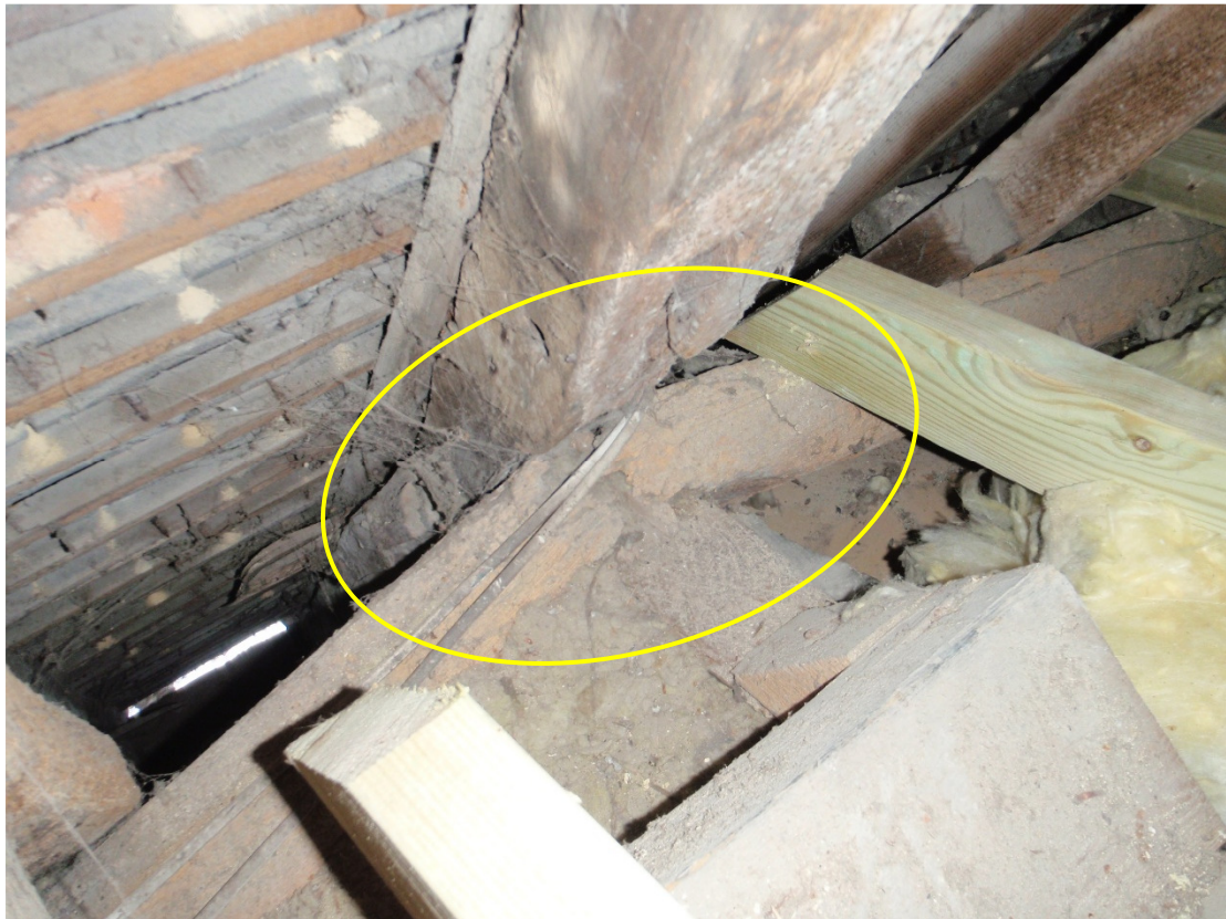
Fig 3 Fractured purlin at truss tie, east side of roof.
