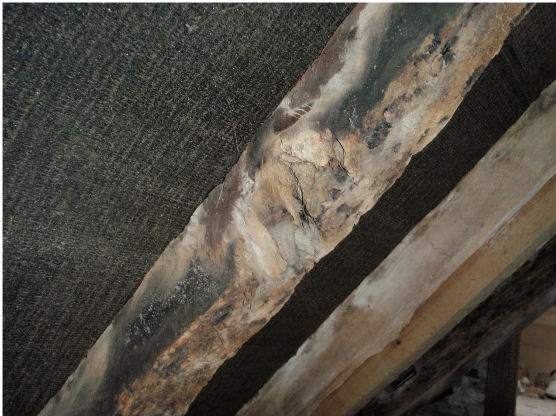
Fig 8 Significant weakening of rafter due to large knot – west slope of roof.
