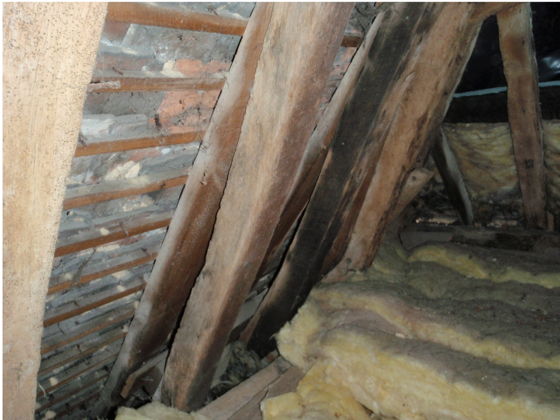
Fig 7 Poor packing to achieve plane slope on east side of roof.
