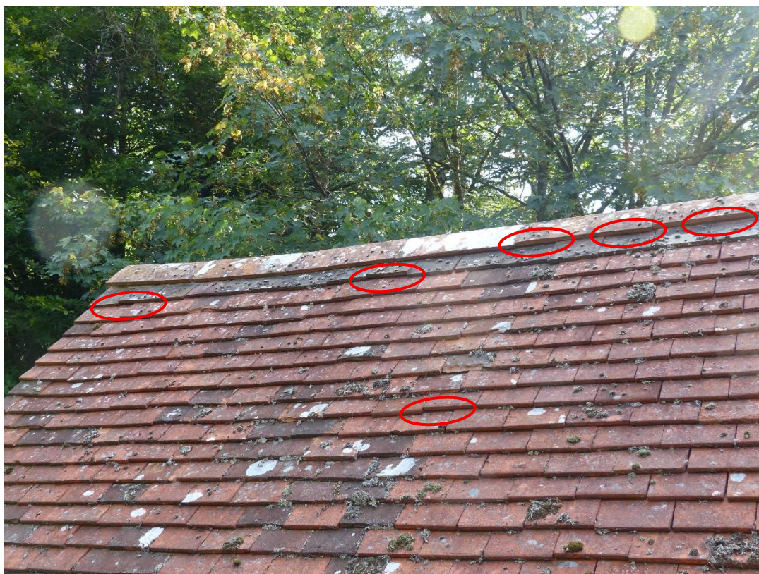
Figure 9 – Gaps below northwestern-facing ridge & roof tiles viewed from flat roof
