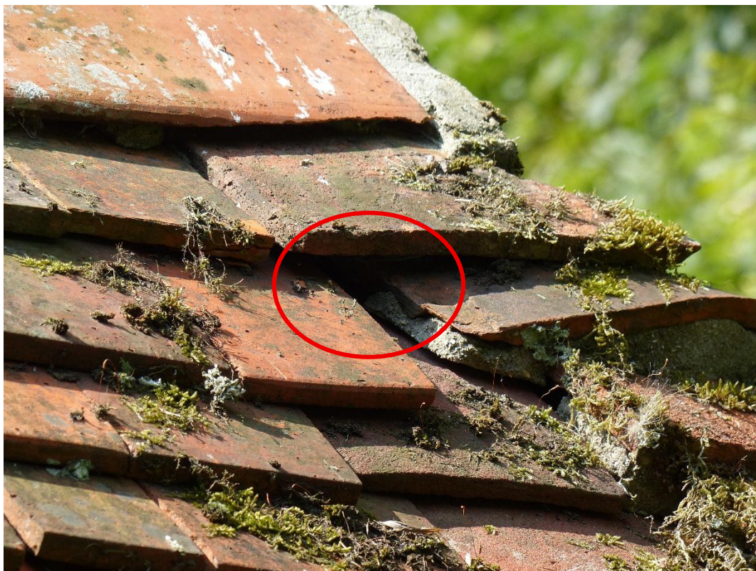
Figure 12 – Missing mortar around bonnet tiles
