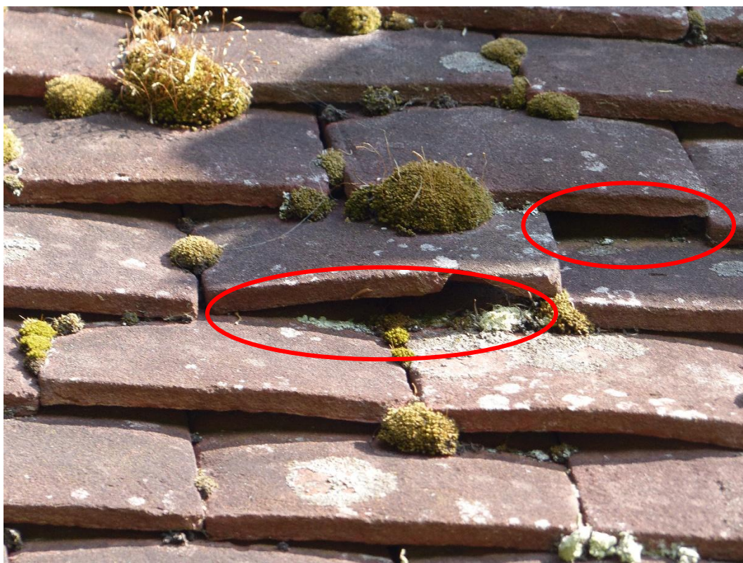
Figure 10 – Multiple raised roof tiles (southern aspect)
