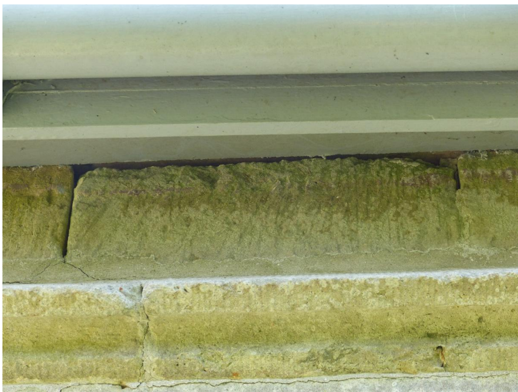
Figure 13 – Gap between soffits & exterior masonry (southern aspect)
