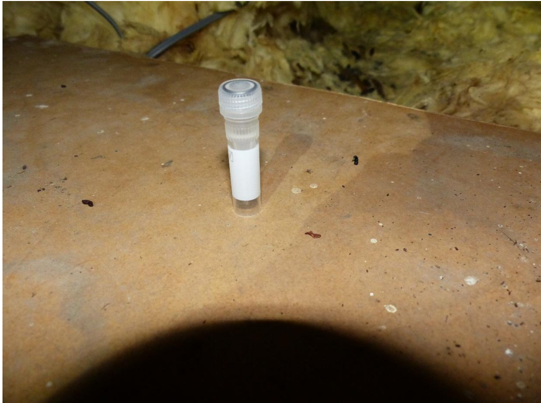
Figure 17 – Common Pipistrelle droppings on northern loft access hatch, with rat & mouse droppings visible on glass fibre insulation
