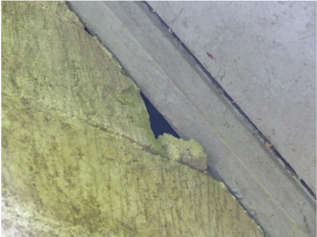
Figure 14 – Gap around stonework on eastern gable
