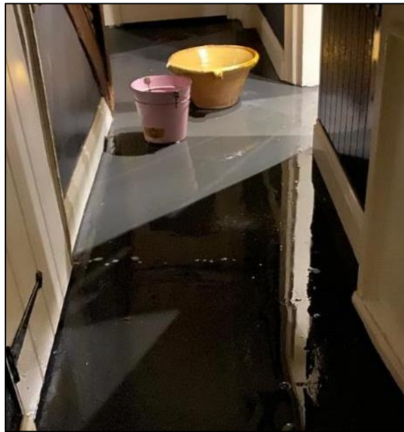
Plate 11. Water damage at the northern end of the ground floor (Mr Craig & Sue Bond, 2025)
