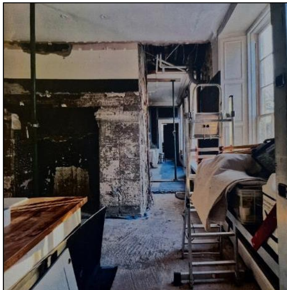
Plate 12. Kitchen chimney breast removed as part of unconsented works
