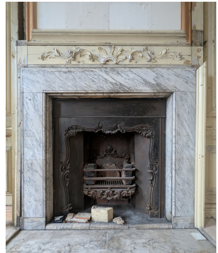
Extant condition, showing missing architrave at top and left hand side, to be reinstated to match that on right
