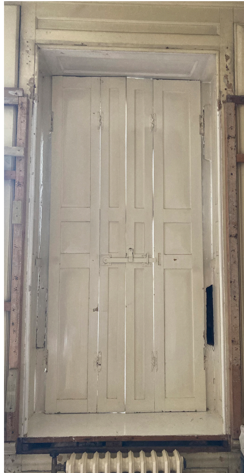
Window with shutters closed, showing locking bar and missing cover to sash box on right hand side
