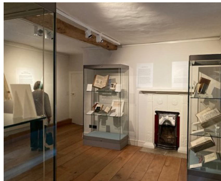
Track lighting (surface mounted): Kelmscott Manor
