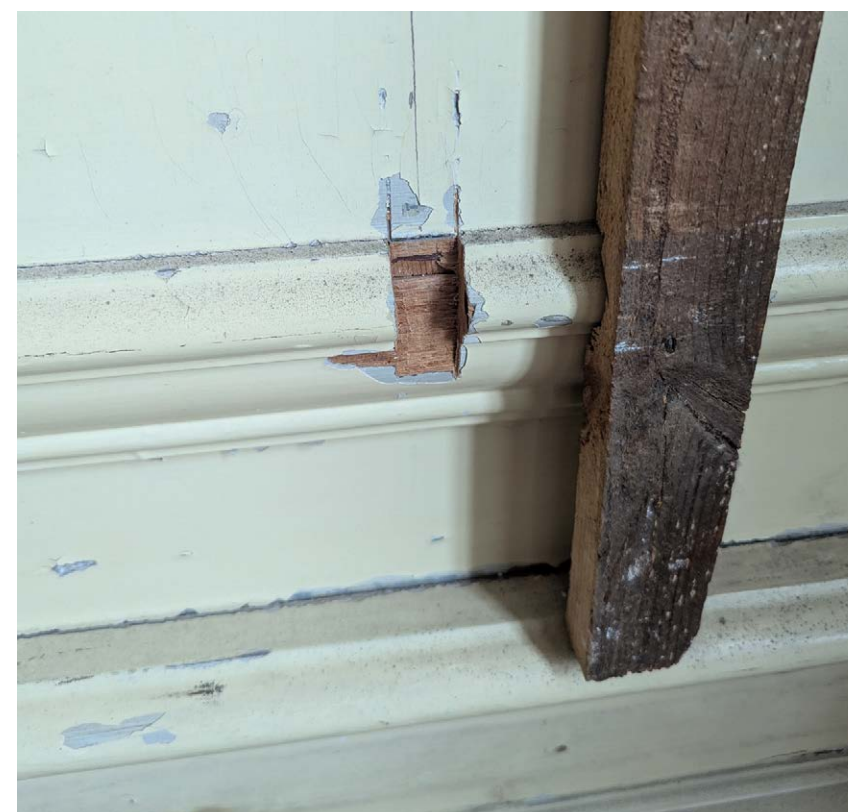
Top: cross-grain shrinkage and loss of connection at panel edge Bottom: localised notching of moulding and loss of fabric
