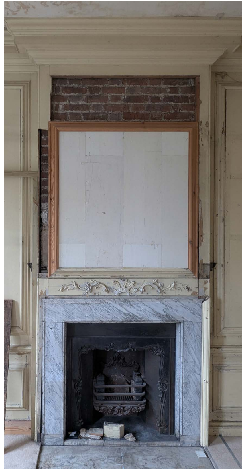
Fireplace, with displaced modern panel above and missing mantle shelf
