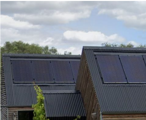
Solar panels Installed in roof finished black
