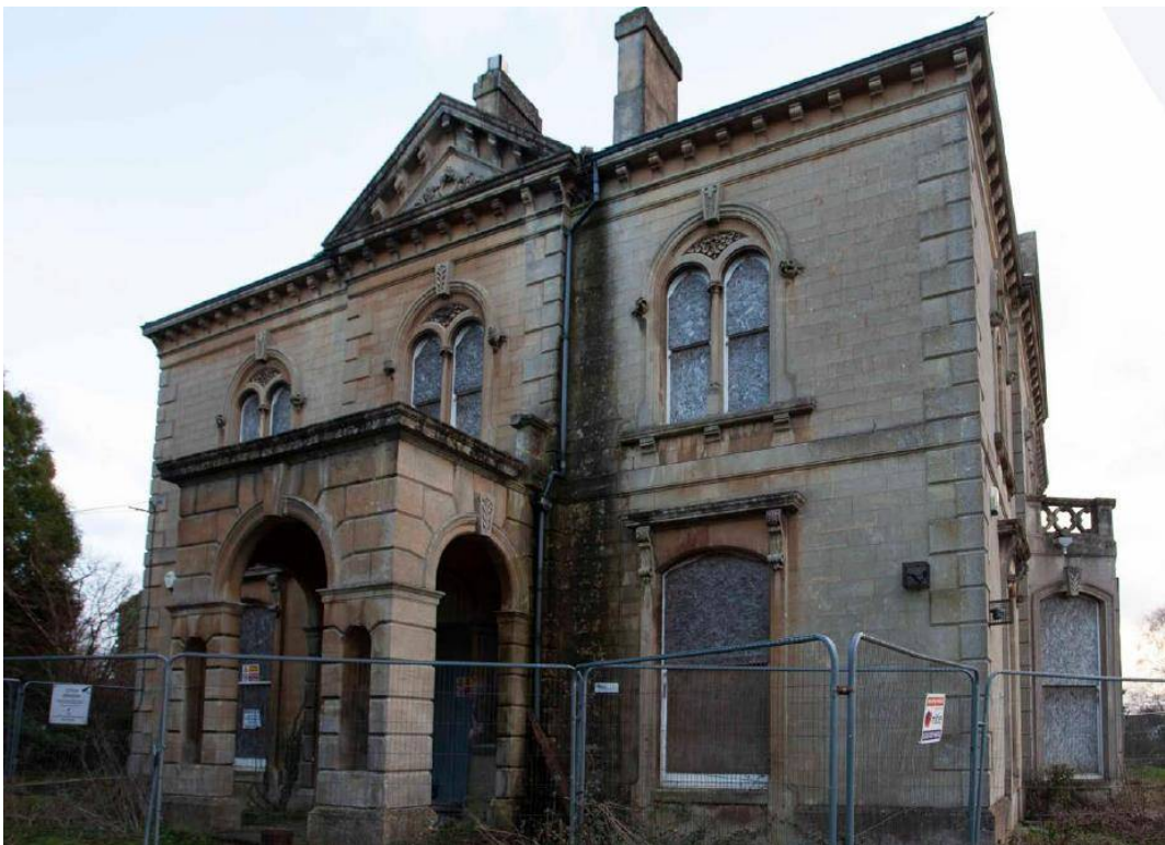
Fig.34 Recent photograph of the front of No.53 – stone balustrade missing from the porch parapet
