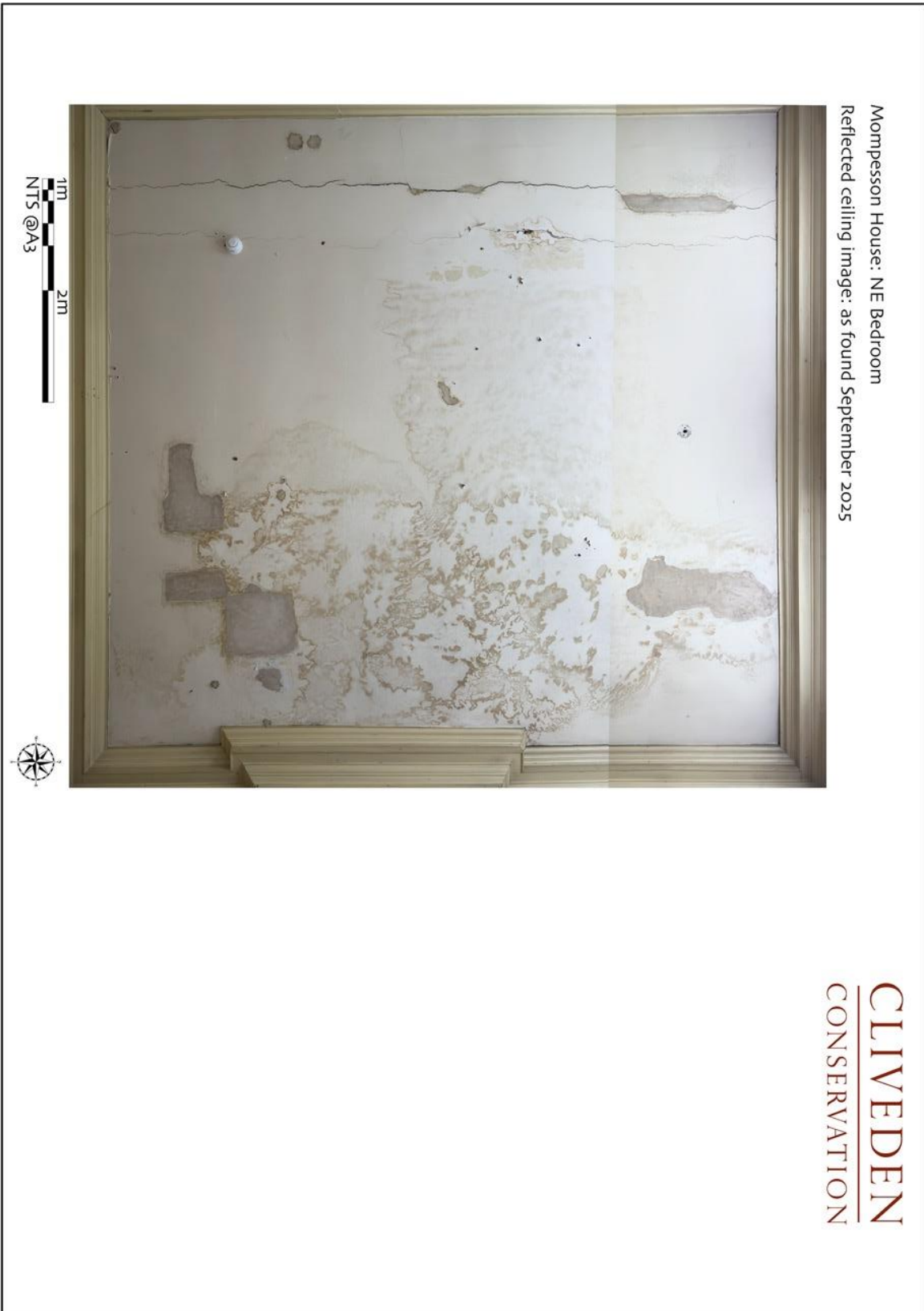
Fig 2: Mompesson House: NE Bedroom ceiling as found September 2025 (CCW/RR)
