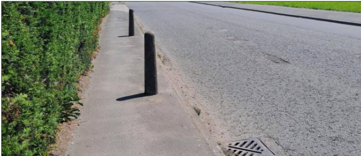
Image 37 - Bollards on Stanier Road
