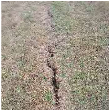
Figure 2-5: Surface desiccation crack present in the south-eastern corner of the site.
