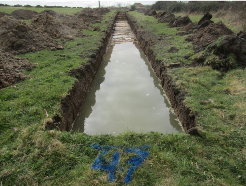
PHOTOGRAPH 3: PARTLY FLOODED EVALUATION TRENCH
