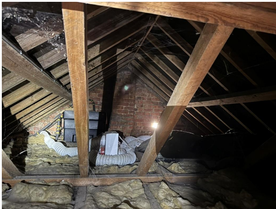
Plate A2: Views towards eastern gable showing hole in wall, with light ingress
