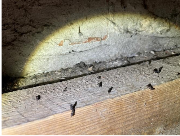
Photo 5 –bat droppings recorded on a rafter in the roof void.
