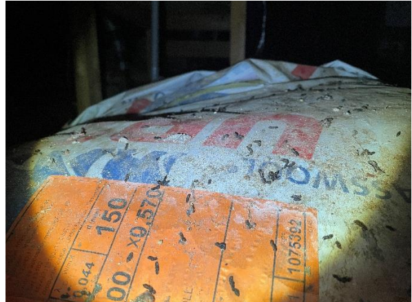
Photo 6 – bat droppings recorded on the floor of the roof void.
