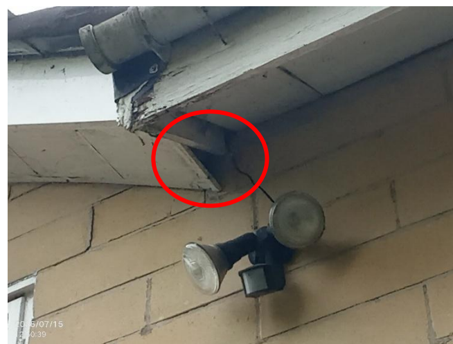
Photo 5: Gap at soffit join.
