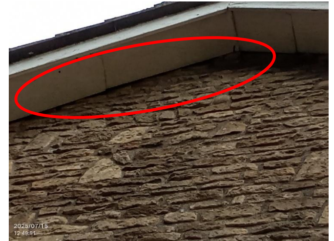
Photo 3: Gaps between soffit and wall top.
