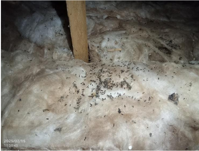
Photo 7: B1 internal bat droppings.
