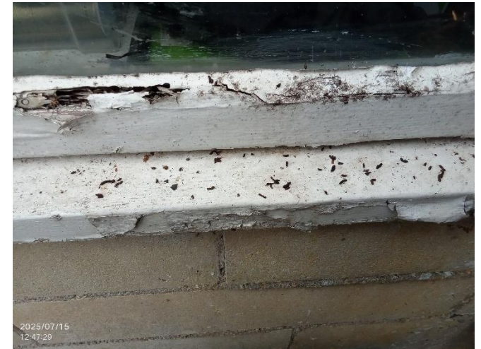
Photo 12: B2 bat droppings on external windowsill.
