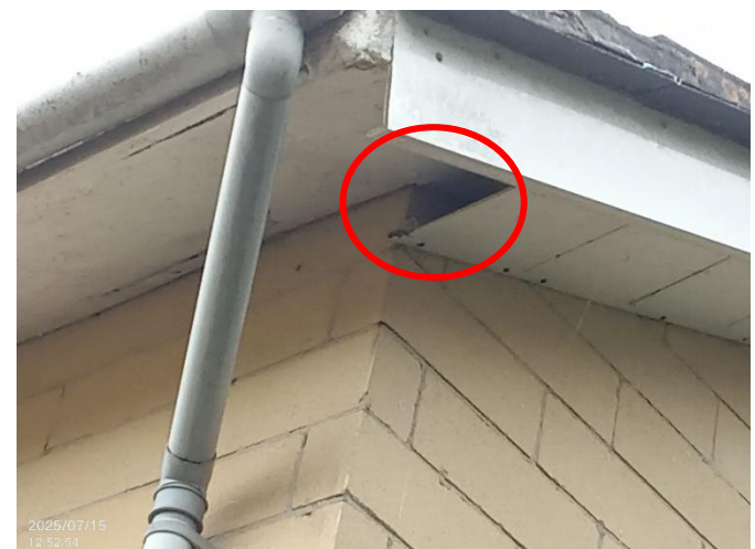
Photo 6: Gap at soffit end.
