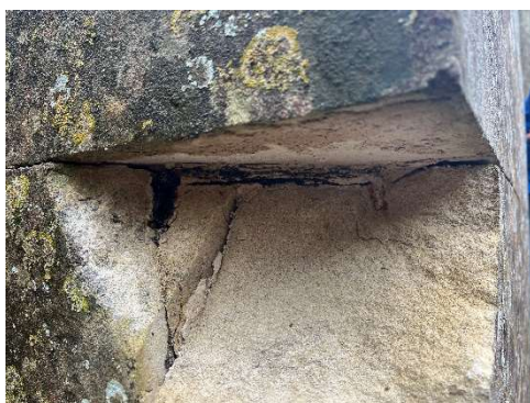
Corroding cramp causing fractures in stone and loss of material.
