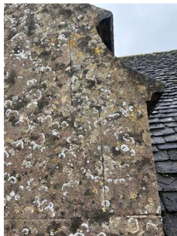
East elevation. Open vertical joints in the stone
