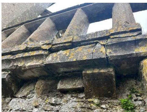
Damaged section of stone below edge of galleried roof to south of inspected chimney.
