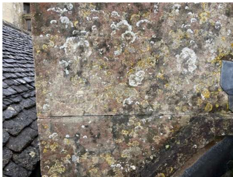
Lower level, north elevation. Open horizontal joints in the stone.
