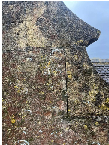
West elevation. Open stone joints leading down to cracked stone.
