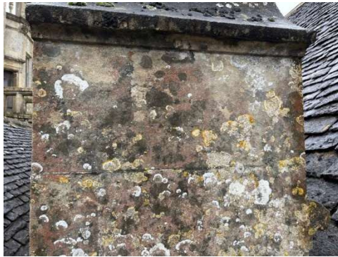
Higher level of base section, north elevation. Open horizontal joints in the stone.
