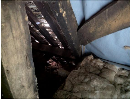
Unfelted rear roof slope with daylight visible in many areas.
