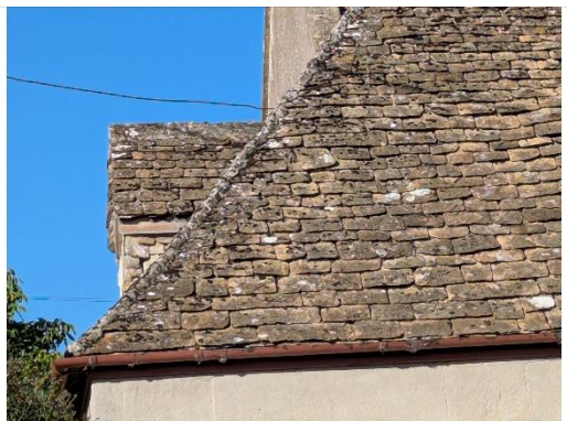
Deteriorated hip detail to the rear right-hand side.
