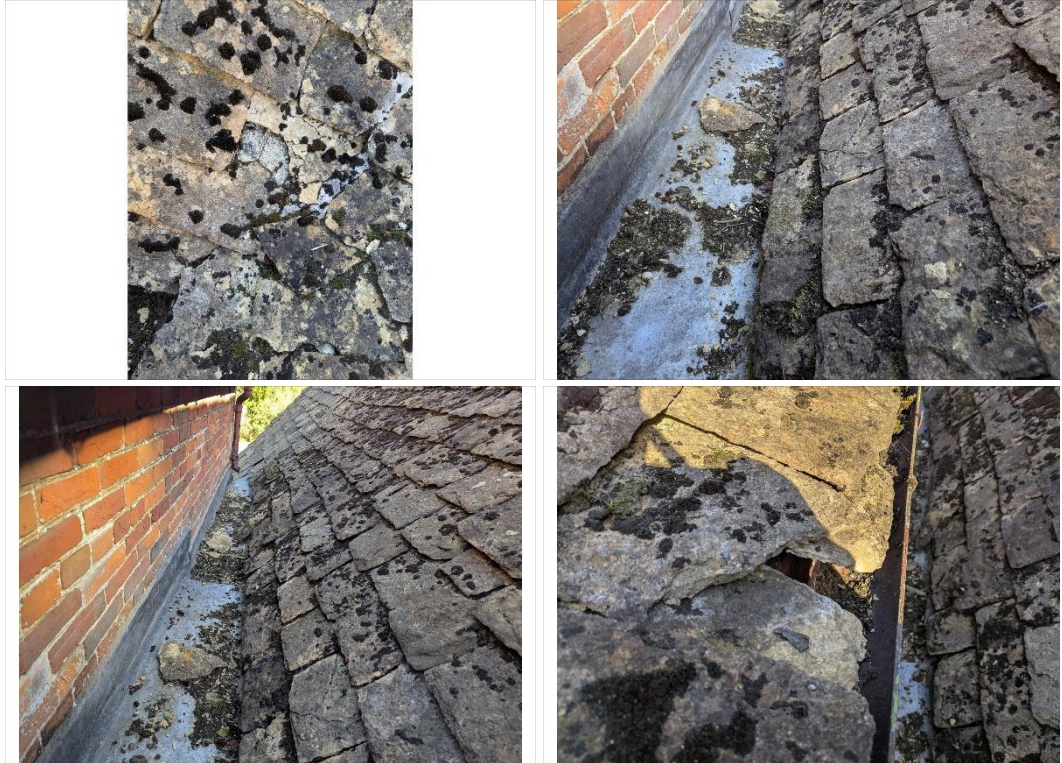
Damaged Cotswold stone slates.
