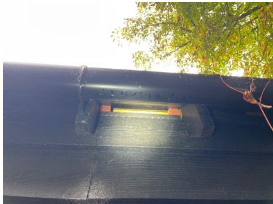
7: Gap at eaves on the east elevation.
