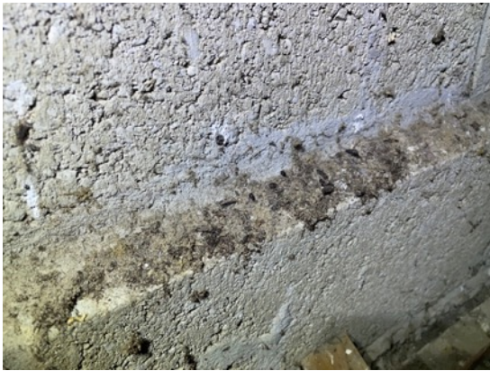
11: Bat droppings on garage wall.
