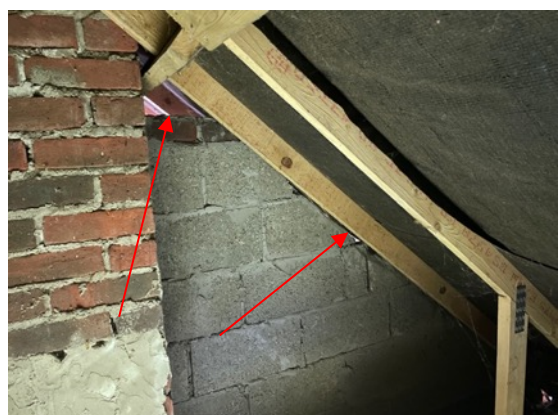
14: Gaps along top of wall providing access from garage.
