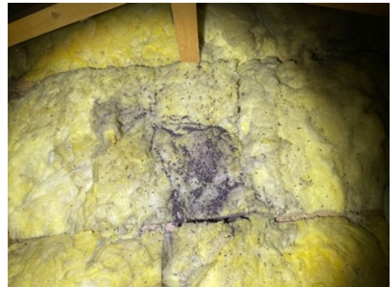
16: Concentration of bat droppings in the south area of the annex roof void.
