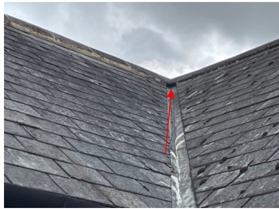
6: Gap at top of northwest roof valley.
