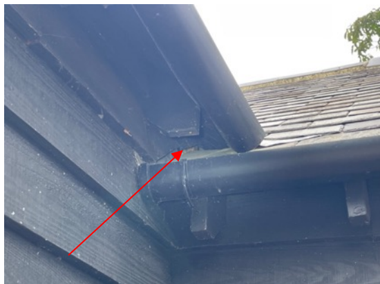
9: Gap at the eaves on south elevation of annex.
