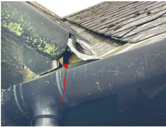
5: Gap at base of northwest lead valley providing direct access to annex roof void.
