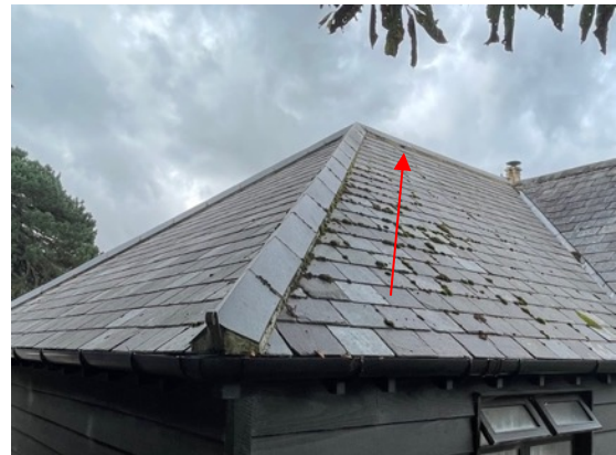
8: Gap in east section ridge mortar.
