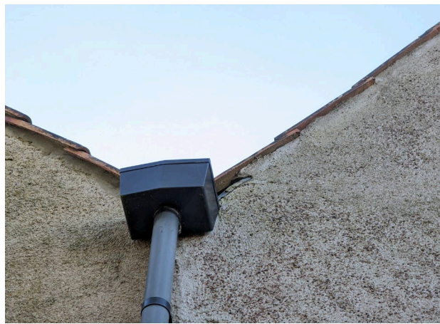
Plate 9: Gap under tile near guttering
