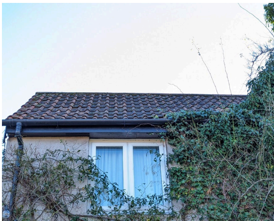
Plate 8: 92 Wood Lane, overgrown ivy
