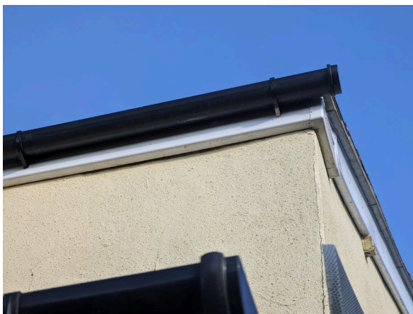
Plate 13: 90a Wood Lane, gaps between fascia board and wall
