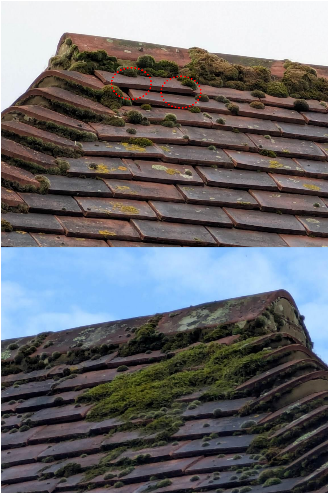
Photo 7/8 Fosbury 40-41 south- west roof tiles with penitential roost access features
